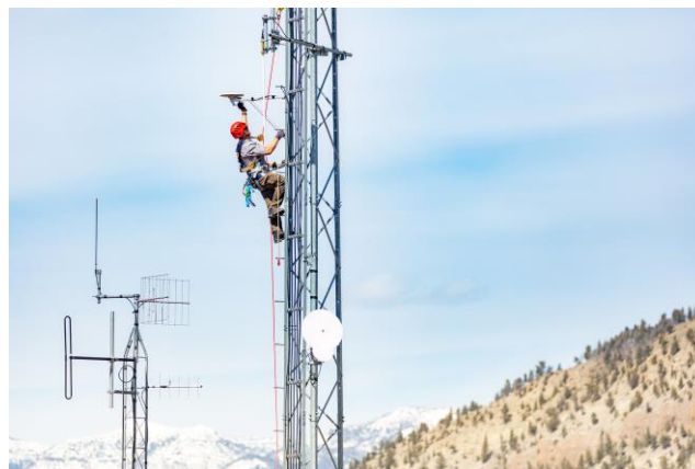
A radio technician works on a tower in scenic terrain in this photo from the job posting. [Photo courtesy of Yellowstone National Park.]
