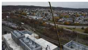
A crane lifts an antenna into place for W3USR's new location. [Photo courtesy of Byron Maldonado, University of Scranton]
